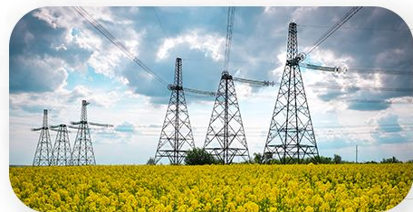
Tubular & Lattice Towers
