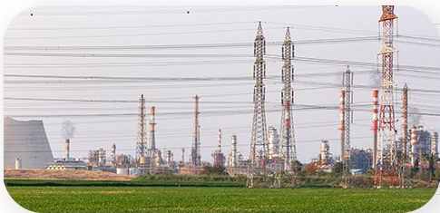
Sub-station Structures for Power Distribution
